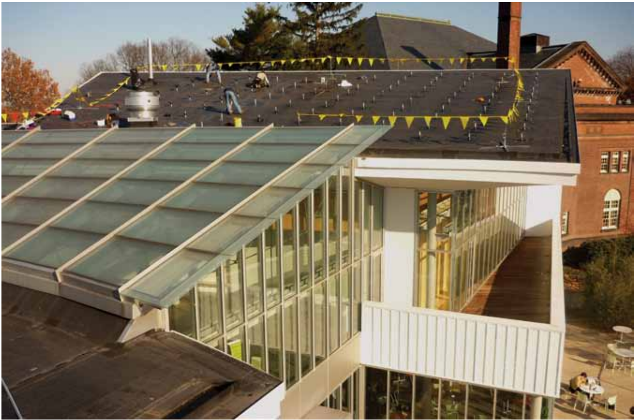
Workers begin the installation of photovoltaic panels on Smith College's Campus Center.
